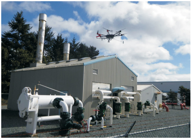
Figure 9. Open-path laser spectrometer on small unmanned aerial vehicle at gas distribution plant in Victoria region, British Columbia.
