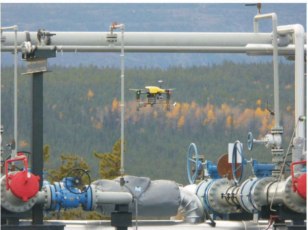
Figure 11. Open-path laser spectrometer on small unmanned aerial vehicle at gas processing plant in Fort St. John region, British Columbia.
